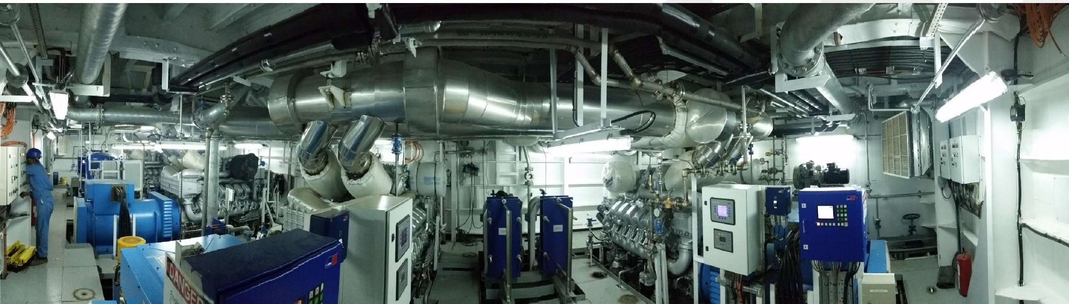
Engine exhaust insulation and cladding
